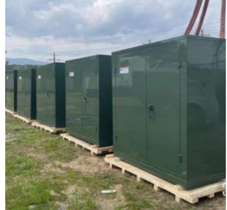
American Electric Power Engineering Project
