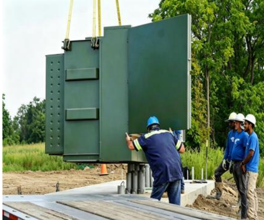
United States Transformer Project
