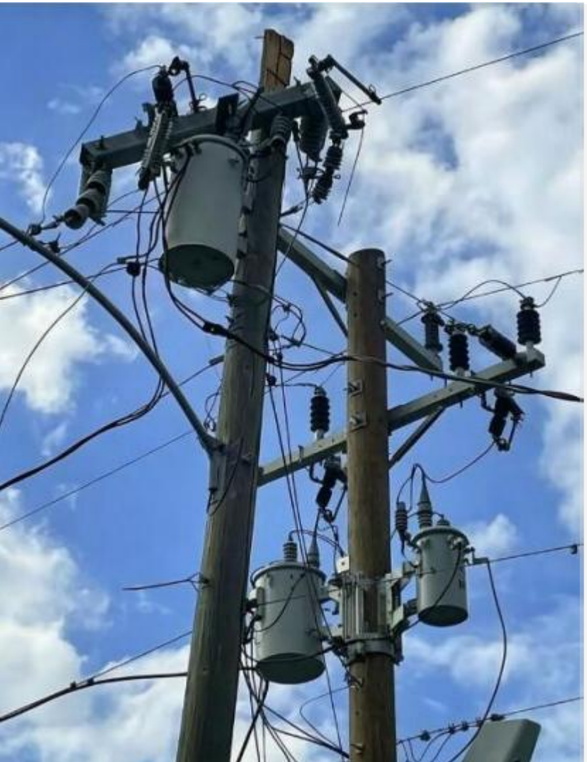
USA Hurricane-Resistant Single- Phase Pole-Mounted Transformer Project
