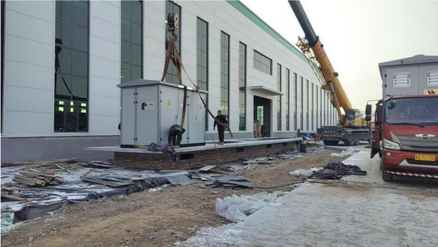
Factory Prefabricated Substation Project
