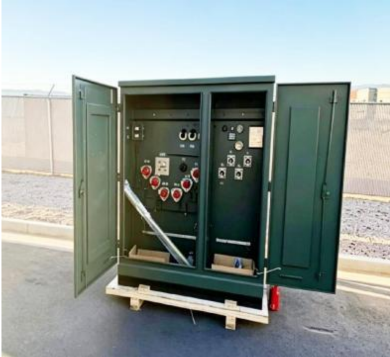
Power Plant Special Transformer
